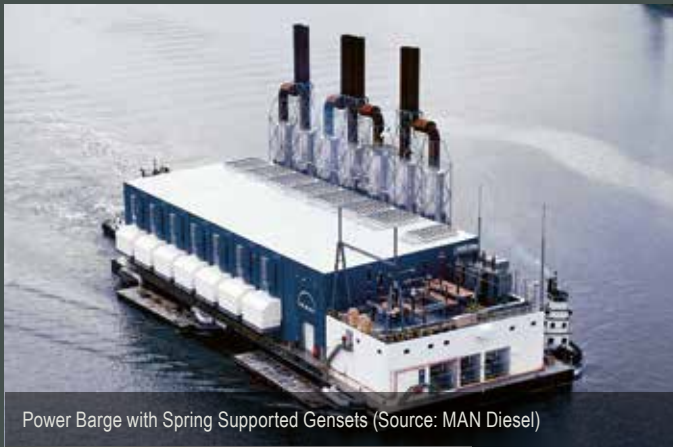
Power Ship with Spring Supported Gensets
